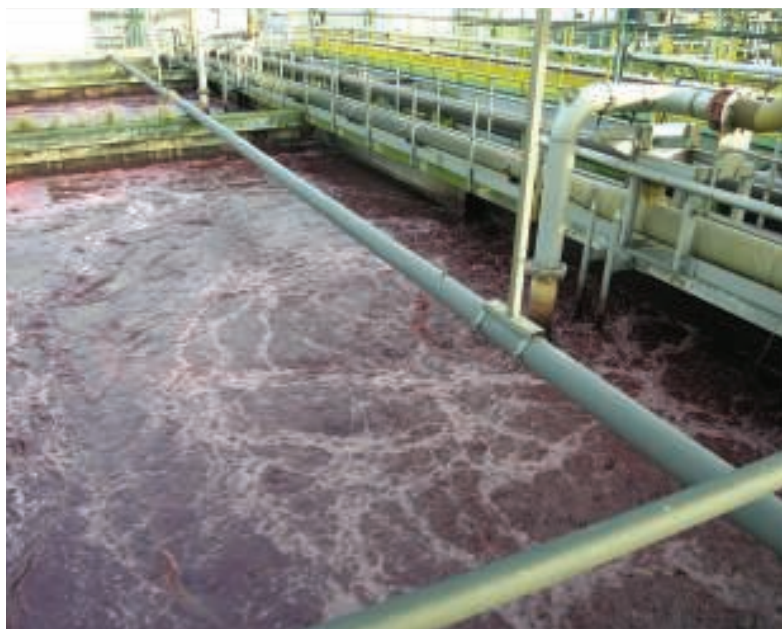
Facility operators often overlook the importance of establishing the right colony of microorganisms in an activated sludge system to target the biodegradable organic pollutants at hand
