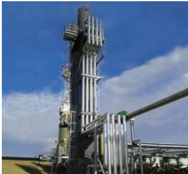
ZEECO Waste Heat Recovery Thermal Oxidizer
